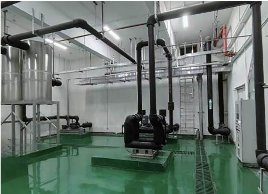
Rainwater and Condensate Recovery System
