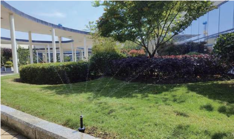
Automatic Green Space Irrigation System
